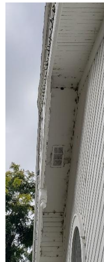
Venting at the original barge rafters.
