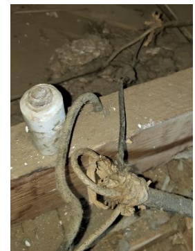
Knob-and-tube wiring seen in the bell tower.
