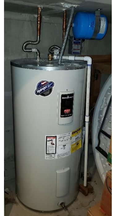
Water heater and expansion tank in the 2000 addition basement.
