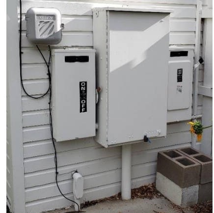
Electrical equipment on the south side of the 2000 addition.
