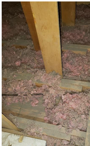
Ceiling joists of the 1941 addition are spliced mid-span and unsupported.
