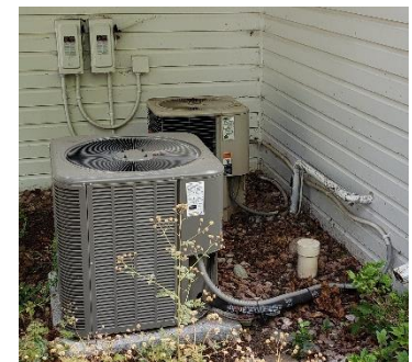
Separate heating and air conditioning for the 2000 addition.
