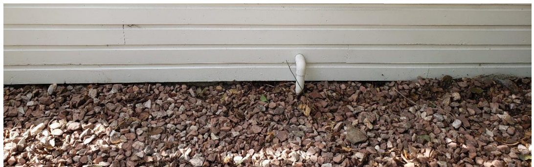
Finish materials sit at grade making it difficult to determine the top of foundation relative to grade.
