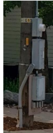
Electrical meter mounted on pole.
