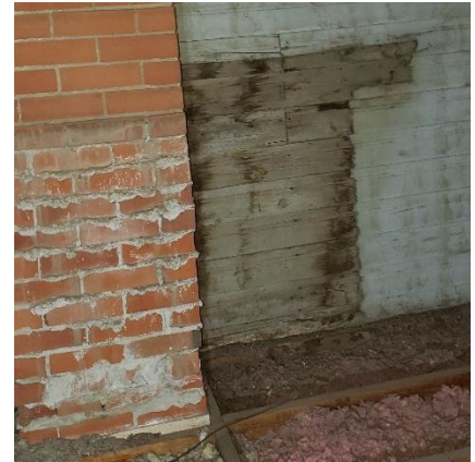
Ghosting of west room seen in the attic.
