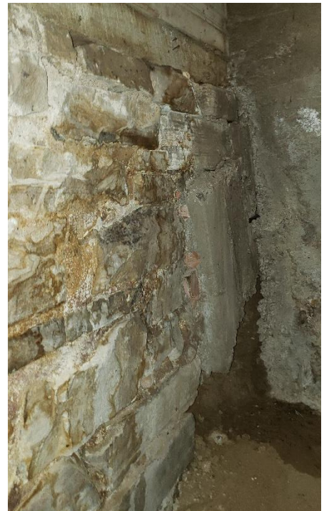
Original stone foundation at basement access area. Water was observed in the basement during a rainstorm.
