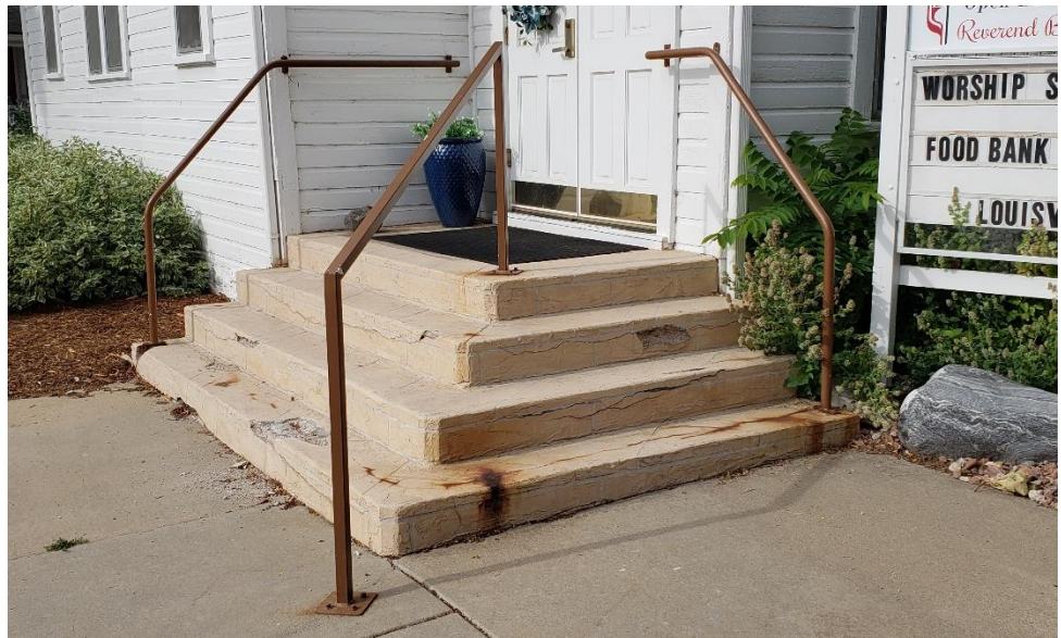
Stairs to the front entrance are cracked throughout and beyond their expected lifespan.
